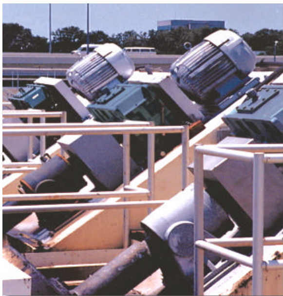
Water Treatment Applications
